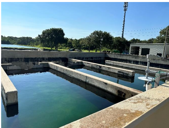
Chlorine Contact Chamber
