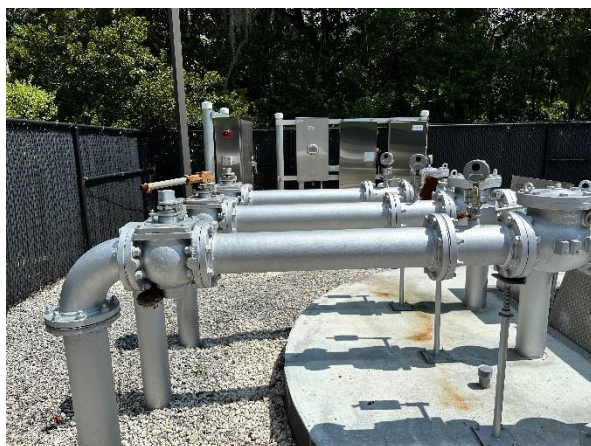
Master Lift Station 1
