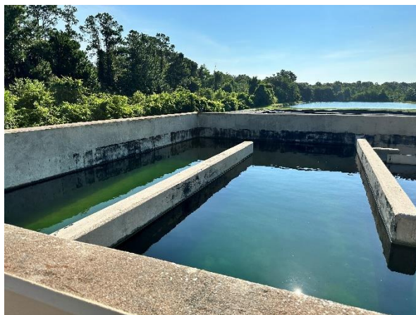
Chlorine Contact Chamber
