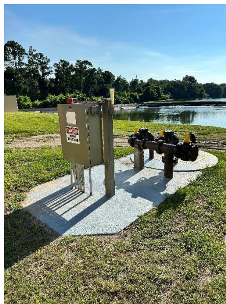
Reject Pump Station
