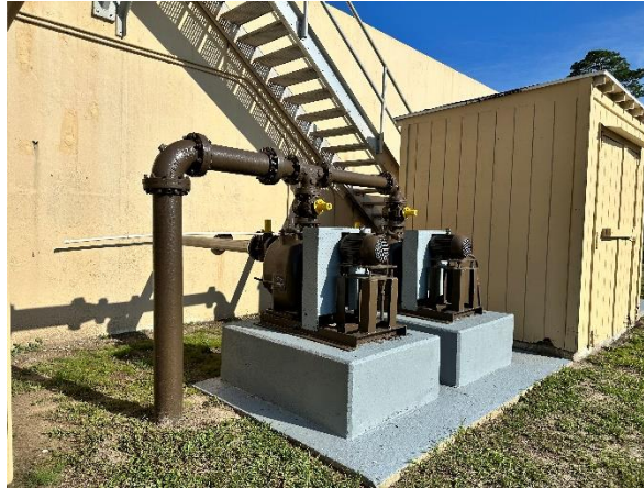
Surge Tank Pumps
