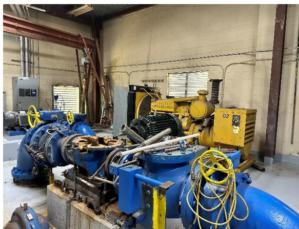
High Service Pump # 1
