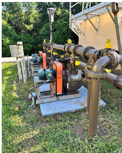
Return Activated Sludge Pumps
