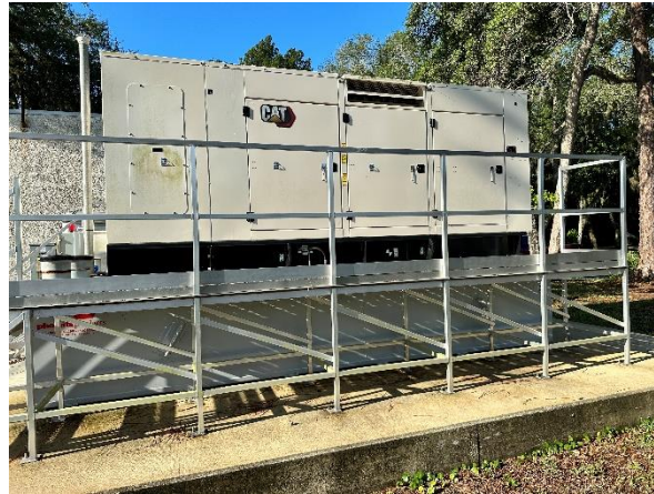
WTP Emergency Generator
