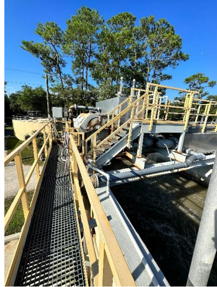
Influent Control Box
