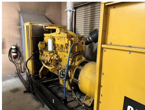
WWTF Emergency Generator
