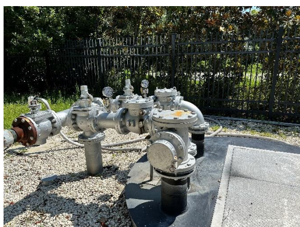
Master Lift Station 3
